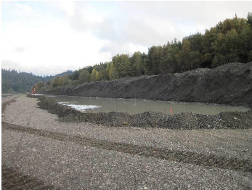
Figure 5. Excavator and trench on Truck Shop Bar during 2012 operations (for example of operations).
